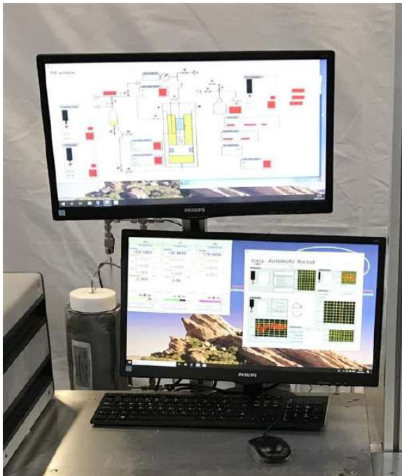
Dual-screen control station — synoptic + acquisition
